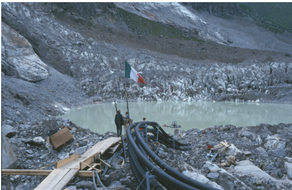
Figure 5.5: Pumps and tubes employed at Lago Effimero, Belvedere Glacier, Macugnaga (Italy) in July/August 2002 (an emergency action in view of the imminent risk of a GLOF from the supraglacial lake which rapidly formed in June 2002 with a maximum water volume of \sim 3.5 million m^3 . In June 2003 a moderately sized GLOF occurred but important damage could be avoided thanks to previous mitigation measures.)
