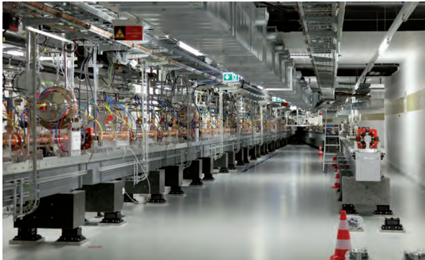
Part of the SwissFEL accelerator complex: accelerating structures for ARAMIS (right) and extraction towards ATHOS (left). More on p. 7.
