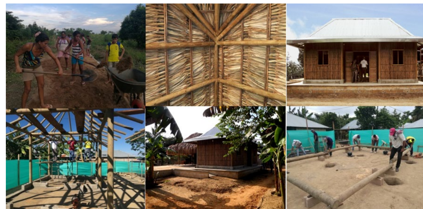
Figure 13. Construction of a modular house in the municipality of San Marcos Sucre with the participation of community members and the use of vernacular techniques (2017)
