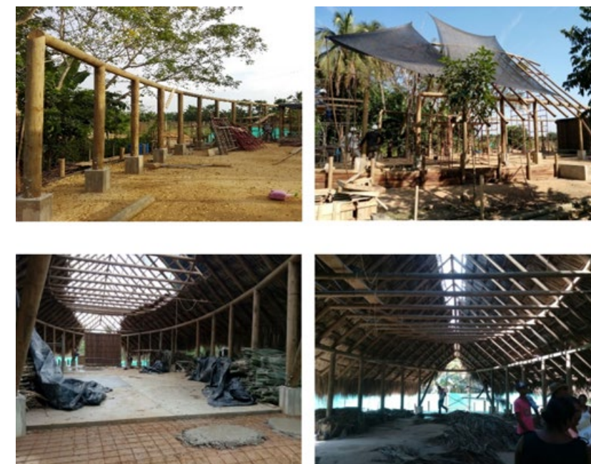
Figure 12. Construction of the community center "El Morrocoy" in the municipality of San Marcos Sucre (2017)
