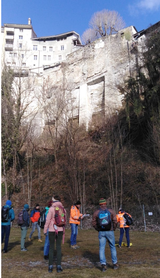
Figure 3: The wall retaining the terrace of the café Le Belvédère partly collapsed.
