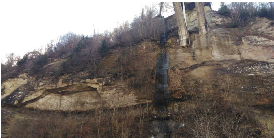
Figure 2: The arch of the Gottéron Bridge rests on a subvertical slope of molasse, without anchors.
